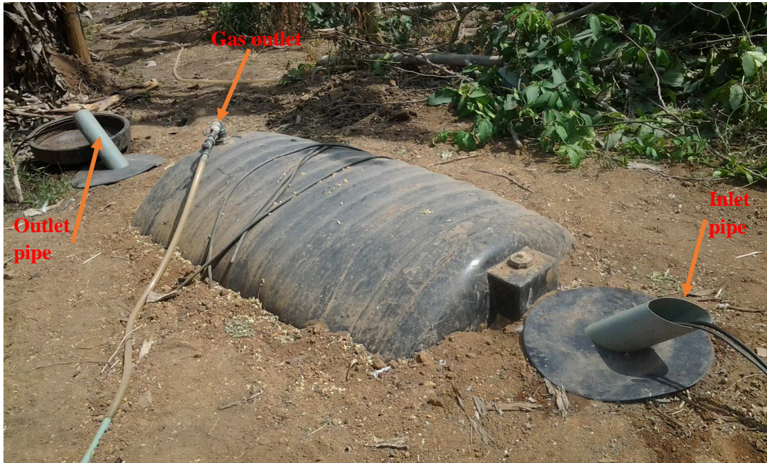
Fig. 1.3: The plug-flow biogas digester equipped with stirrer after installation in a sub-surface pit.
